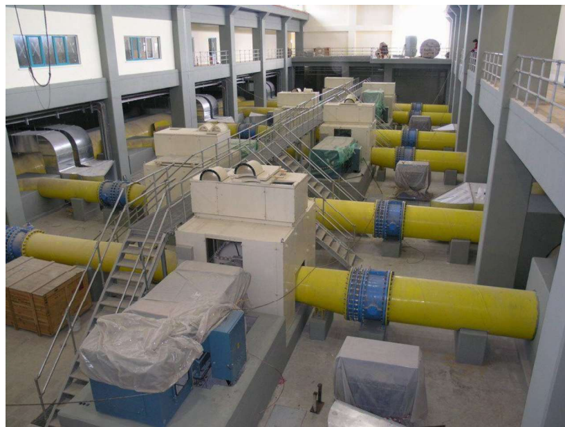
Figure 7. Pumping station in GMP
