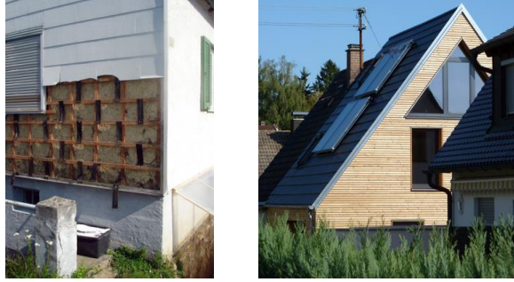
Figure 12: The facade originally contained panels that contained asbestos, but they have been replaced with new wooden panels (Passive House Database, 2023).
