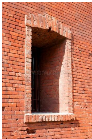
Figure 1: An example of a window being positioned on the inside due to the thickness of the building element in the facade (Dreamstime, 2023).
